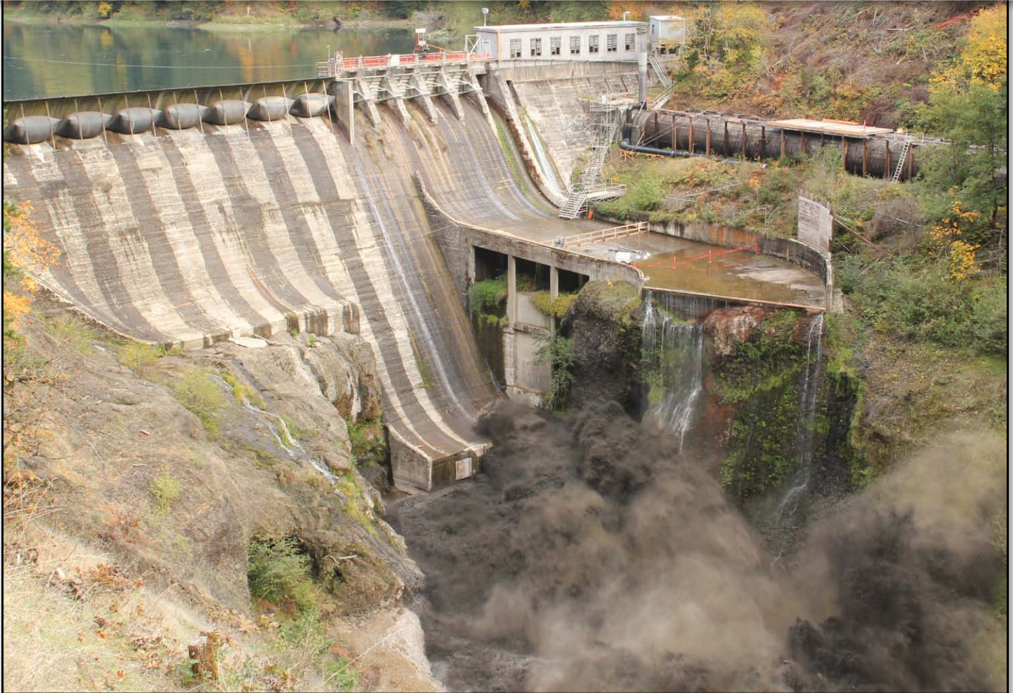
The demolition of Condit Dam; the rebirth of the White Salmon River (WA). Made possible, in part, with your donations Photo: Andy Maser & Steve Stampfli
